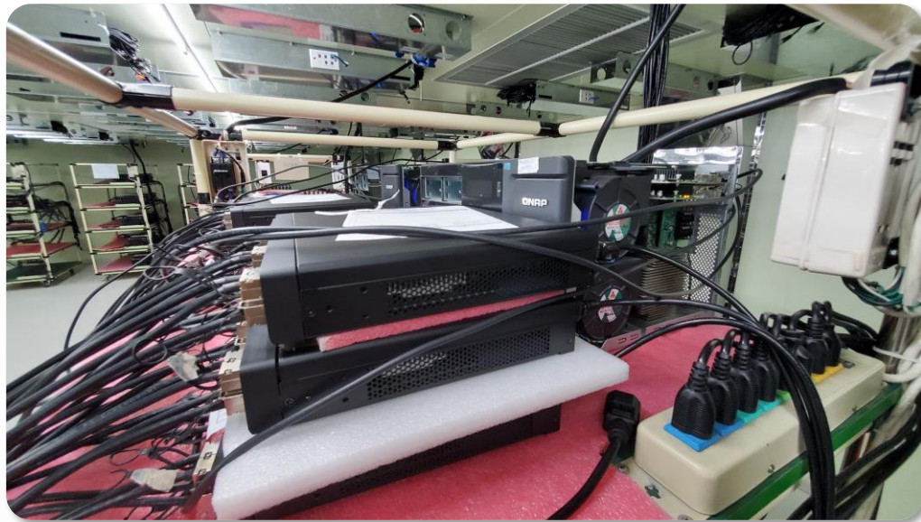
Thermal test equipment and device
